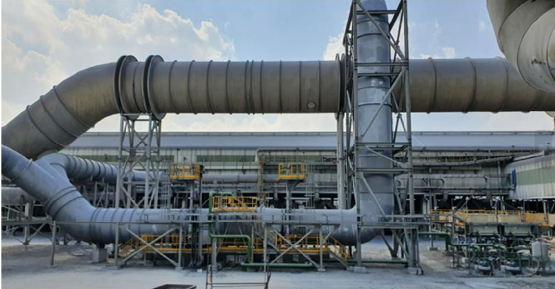
Figure 2. EHEX at Al Taweelah PL 1 East (5311-800). Fumes are collected from nearby pots, cooled, and a mixer (vertical structure) brings it in to the GTC inlet duct (on top).
